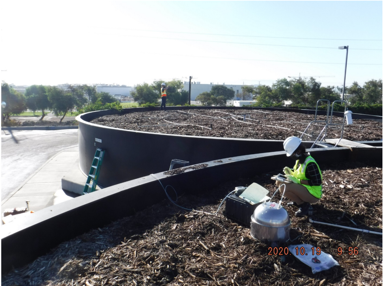
Figure E-1. Vacuum chamber and flux chamber on biofilter surface at ZWED
