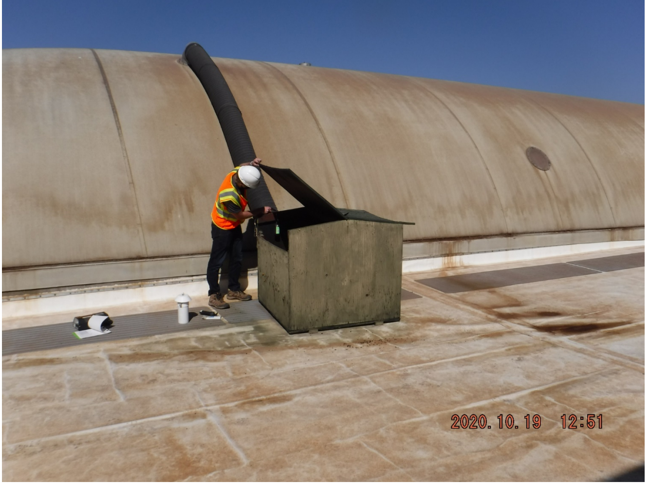
Figure E-5. Carbon filter unit serving biogas bladder at ZWED roof
