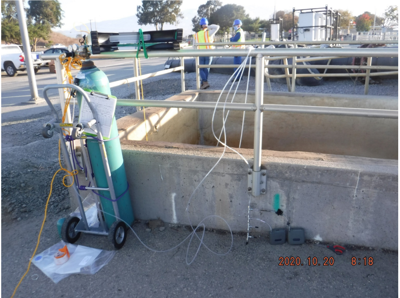
Figure E-7. Nitrogen purge gas cylinder at RWF primary influent channel
