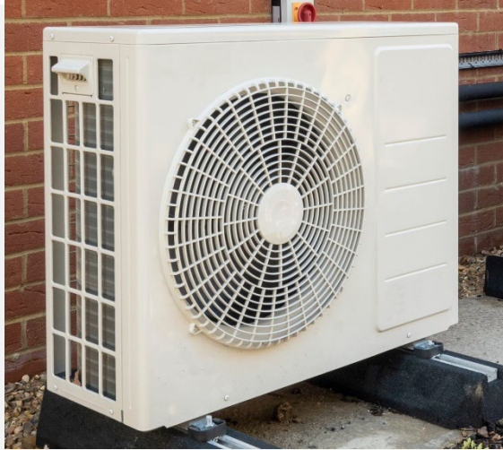
Heat Pump (exterior)
