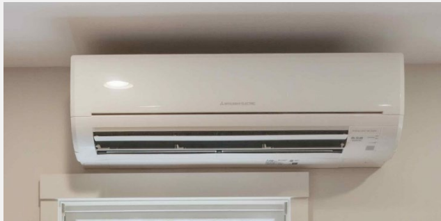
Heat Pump (interior)
