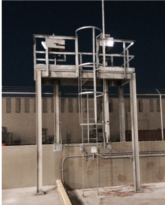
Figure 19. Example of a UV-DOAS analyzer installation on an elevated platform.
