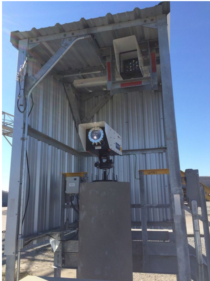
Figure 17. Example of a UV-DOAS analyzer installation.
